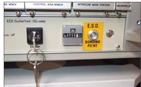
IBAK BG, elapsed hour meter and ESD bonding point
