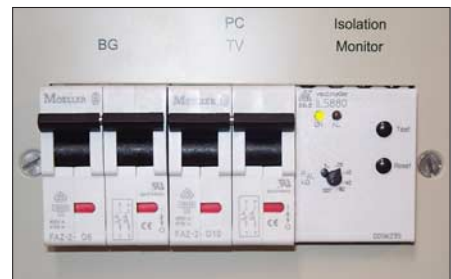
IBAK EV, power distribution panel with automatic fuse and insulation controller
