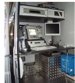
Outfitting operator's section
